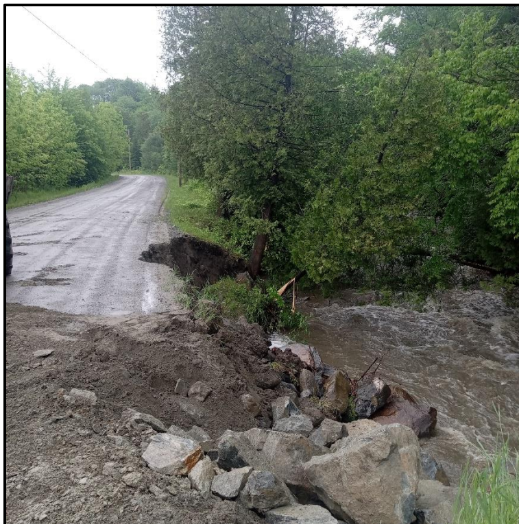
Figure 5: Localized damage to Stannard Brook Road and bridge in the town of Stannard, VT due to heavy rainfall on June 17, 2023. This was the only report of flood damage in the NWS Burlington HSA during the month.
