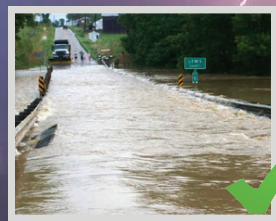
Road Impassable/Traffic Impacted/Cars stranded. ✓
