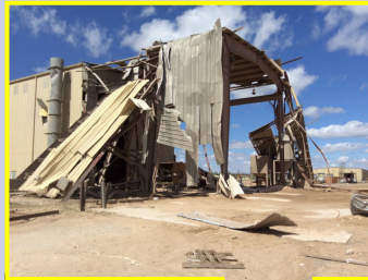
Left: One of several metal buildings damaged near Tulsa International Airport. This was the only area within the 20 mile path where EF-2 damage was found.
