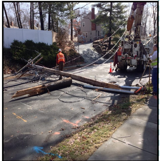
Above: Downed Utility Pole in Brookline, MA - Photo by: KB1NCG-Marek Kozubal
