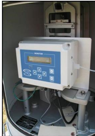
Figure B-20. FPR-D Data Logger
