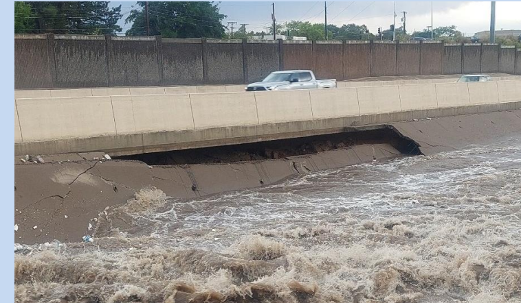
ABQ I-40 Arroyo Flood | August 8, 2023 Courtesy NMDOT
