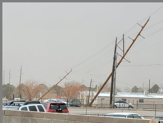
Damaged Power Poles | ABQ Courtesy Susan Cessac
