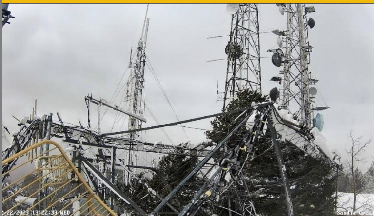
Sandia Crest Damage | February 22, 2023 Courtesy Jeff Burmeister
