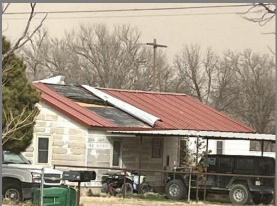
Roof Damage | Hagerman Courtesy Hagerman PD
