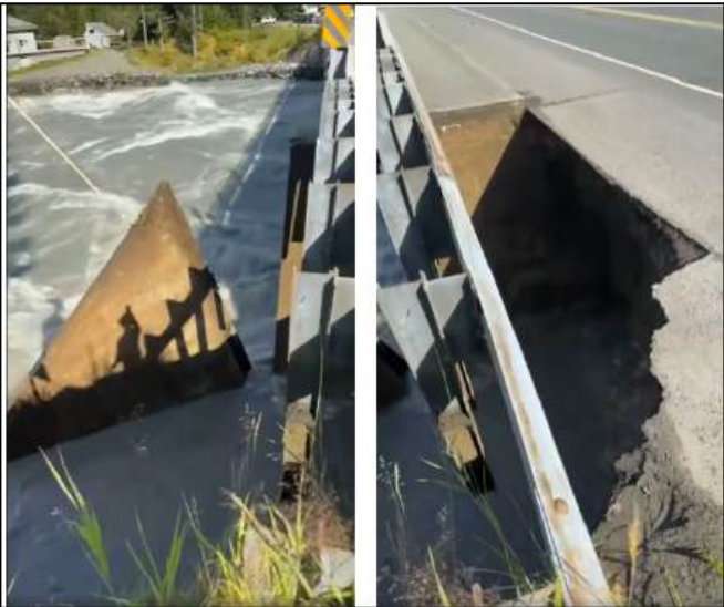
Image 2: Damage to Back Loop Road Bridge and a telecommunication/power pole. Photo courtesy of NWS.
