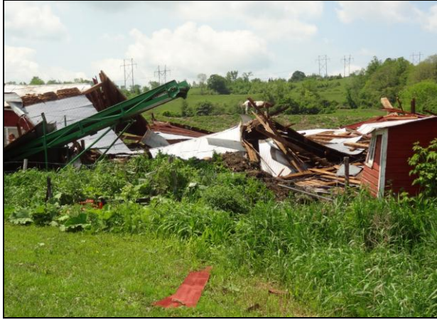
Figure 1: Barn destroyed at the corner of Bernaski Rd. and NY Route 30. This barn was over 100 years old.
