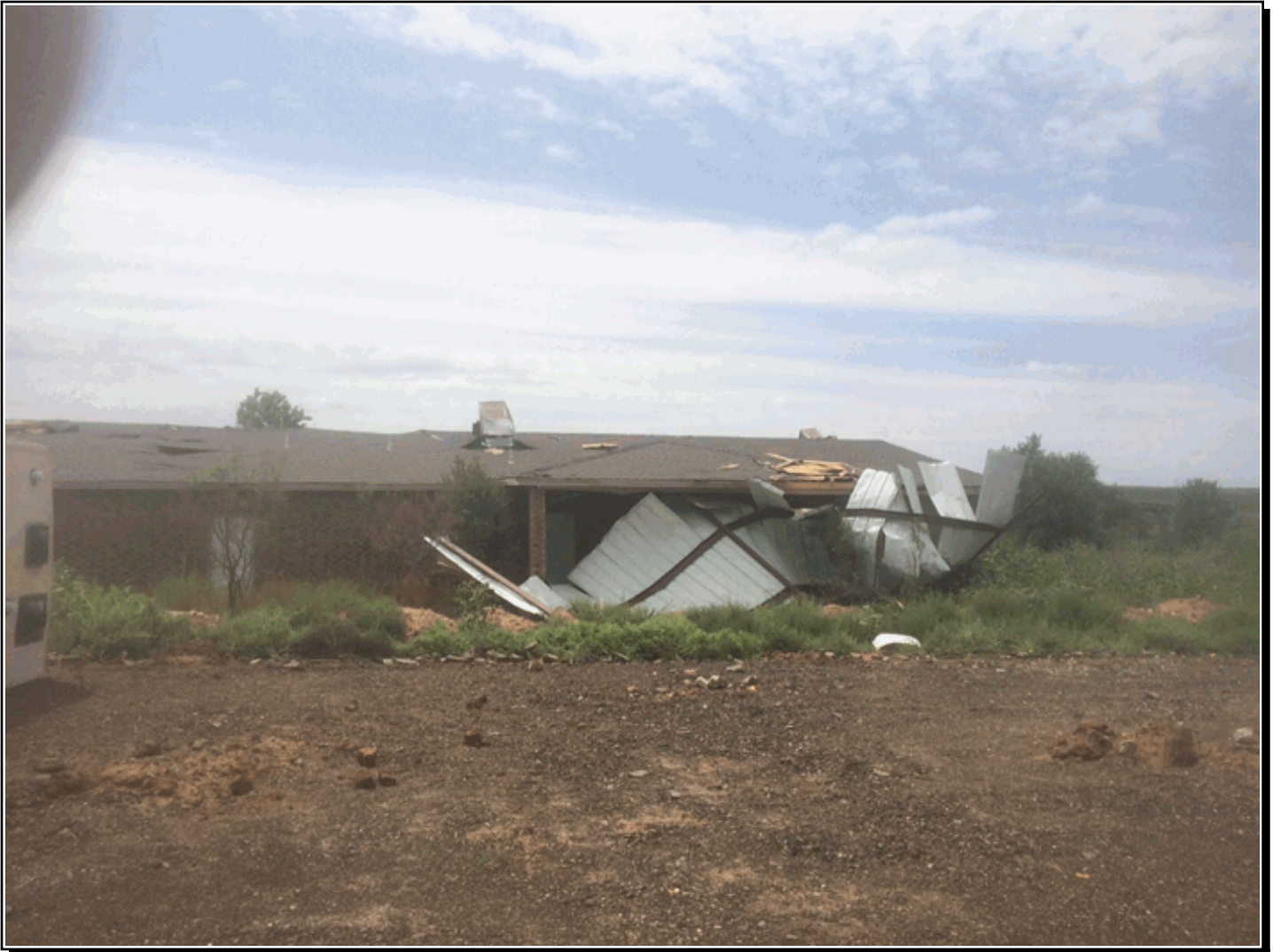
Thunderstorm wind damage near Loop 335 and Hester.
