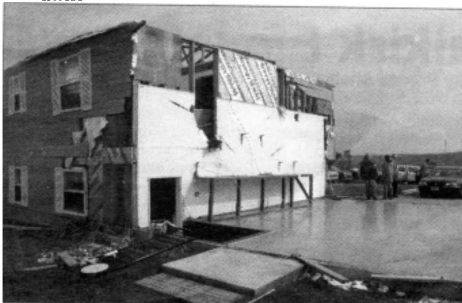
A two story farm house about 9 miles southwest of Underwood, North Dakota, with the garage completely torn away and the roof gone after an F2 tornado on August 24, 2006. Photo by Cory Neumiller and courtesy of the Underwood News newspaper.
