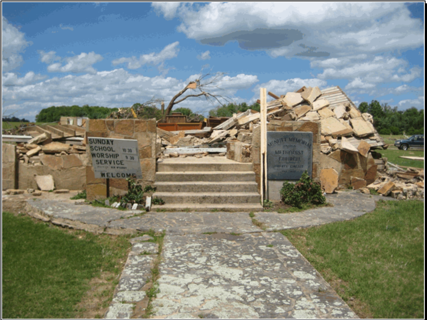
An EF-4 tornado destroyed the McNutt Memorial Methodist Church in DeKalb County.
