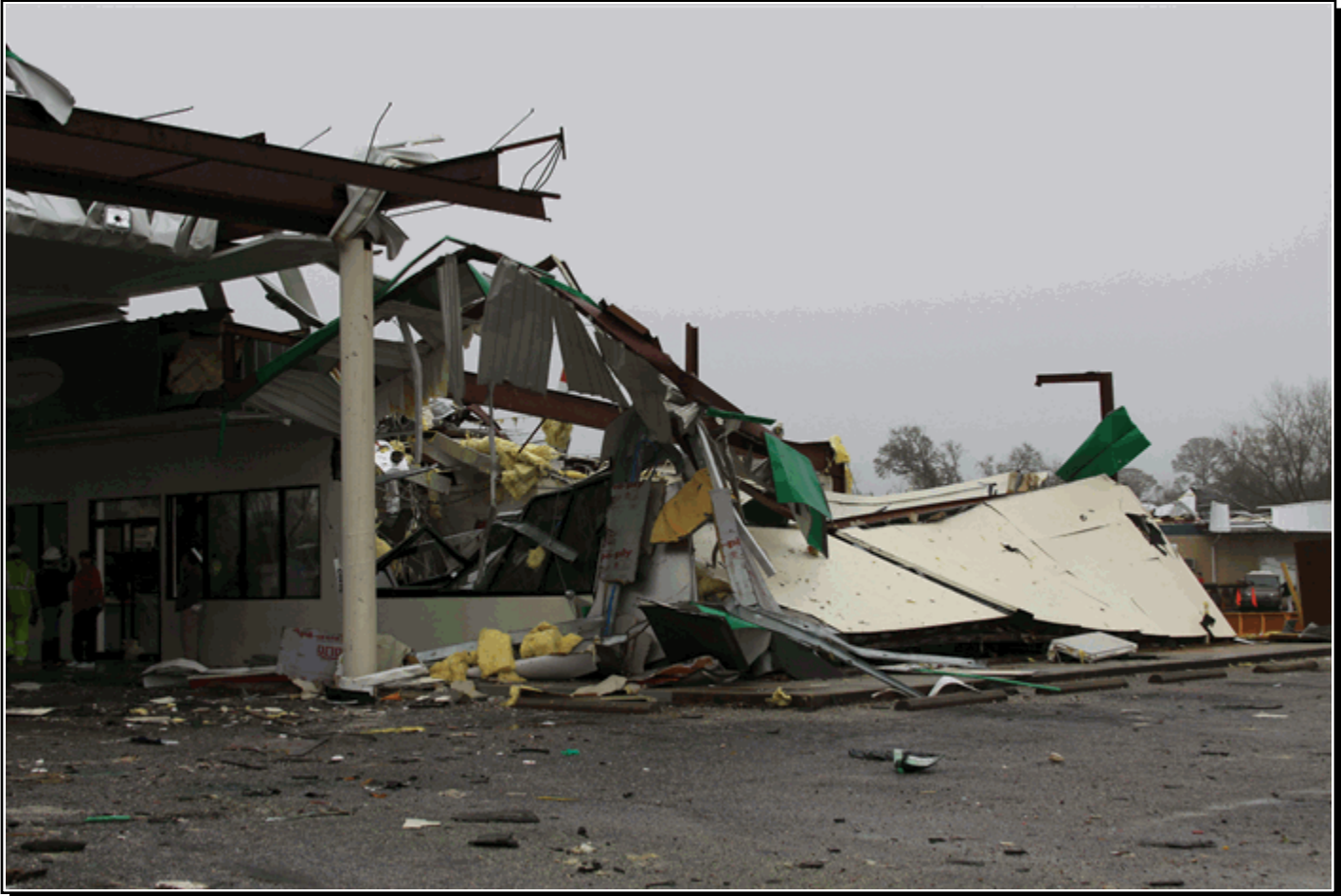
BP convenience store destroyed as the EF-2 tornado moved through. There were 4 injuries at this location.
