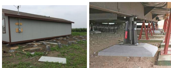
Figure 10. One example to improve resiliency: Anchoring a mobile home. At left, this home slid off cinderblock piers with no anchors. At right, a pier/anchor system for home that would likely withstand low-end hurricane-force wind.
