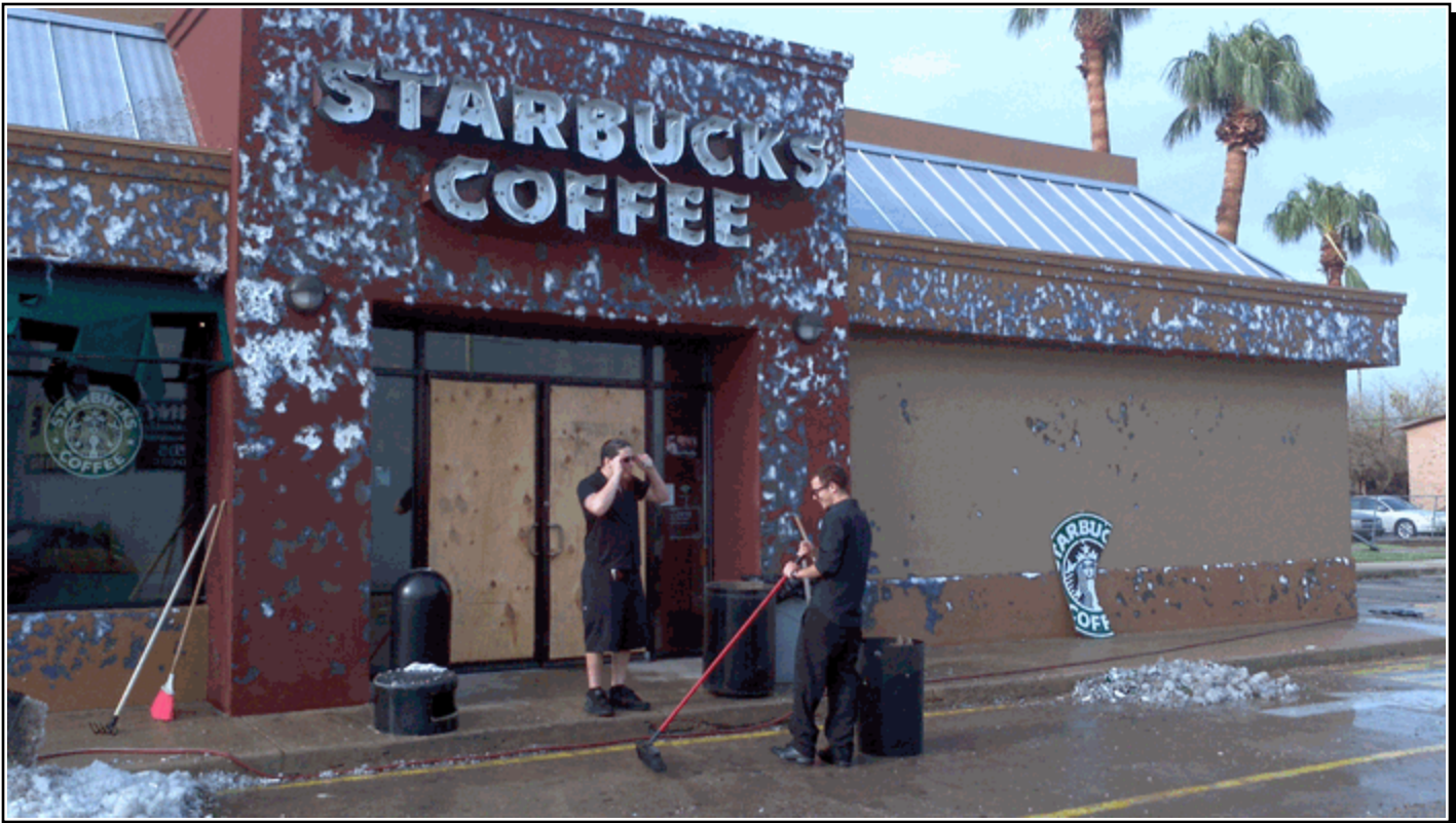
Building damage due to wind and hail in McAllen.
