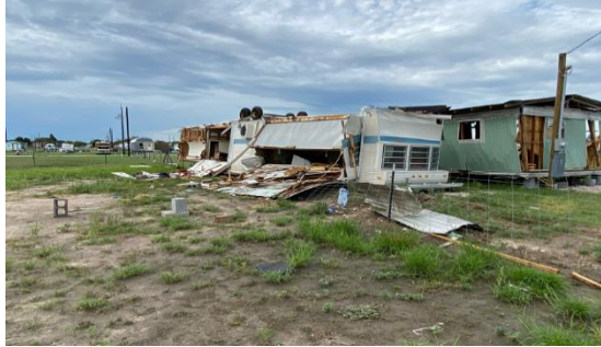
Above: Flipped, unanchored trailer destroyed by estimated 75 mph gusts in San Carlos, TX (east of Edinburg), in the wake of Hurricane Hanna in late July 2020.
