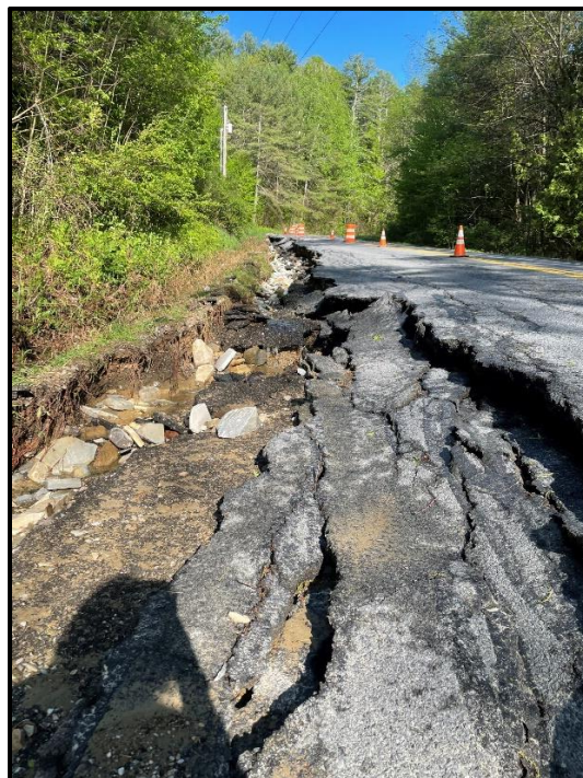
Figure 2: A roadside washout in the Town of Proctor, VT. This was the result of torrential rainfall and localized flash flooding on the evening of May 16, 2022.
