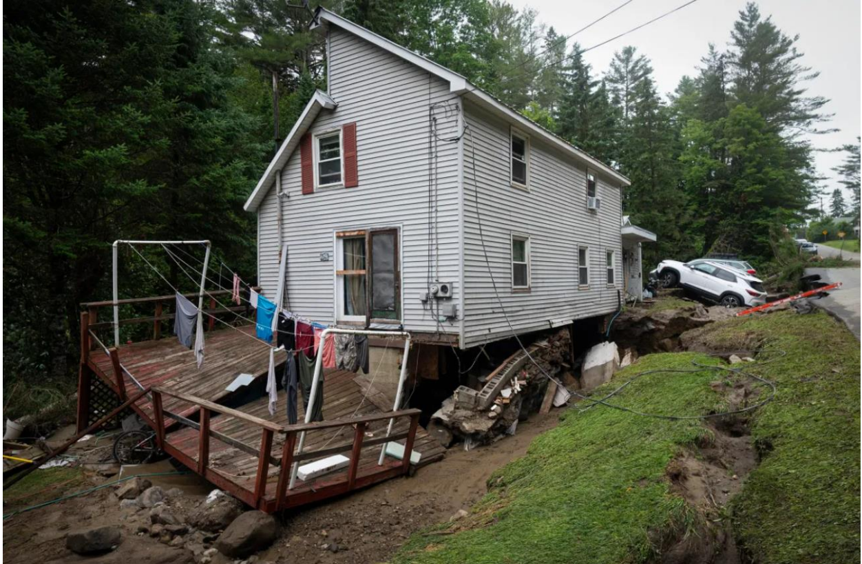
Figure 6: Photo of flash flooding damage to a home on Calendar Brook Rd provided by VT Digger.
