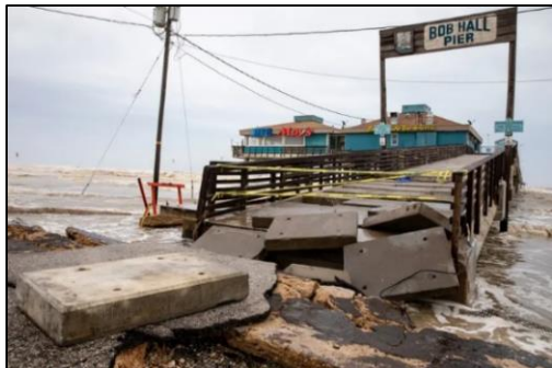
Damaged entrance to Bob Hall Pier. Image – Courtney Sacco
