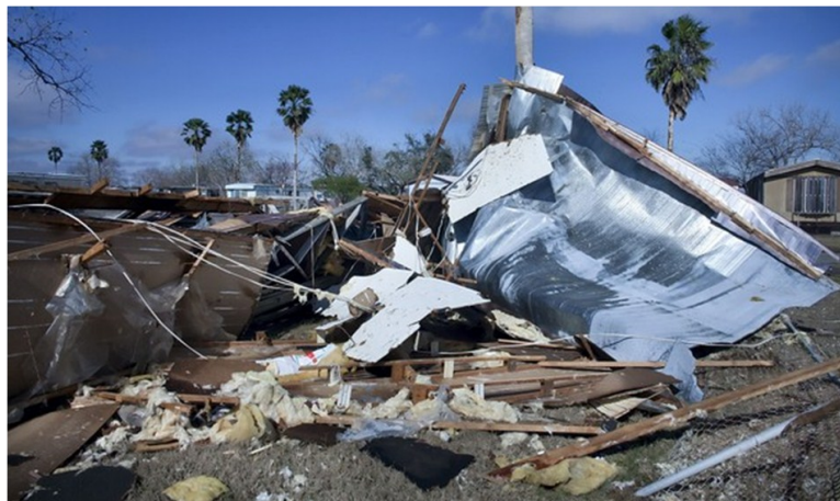
(Right) This mobile home in Portland was completely destroyed by the strong straight-line winds.
