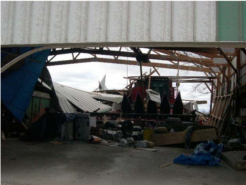
Machine shed roof damage near H Ave. northwest of Pilot Mound in Boone county.
