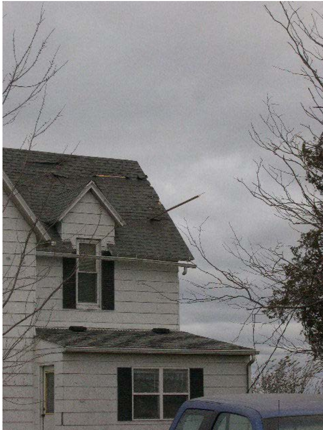
Board embedded through roof of home near H Ave. northwest of Pilot Mound in Boone county.
