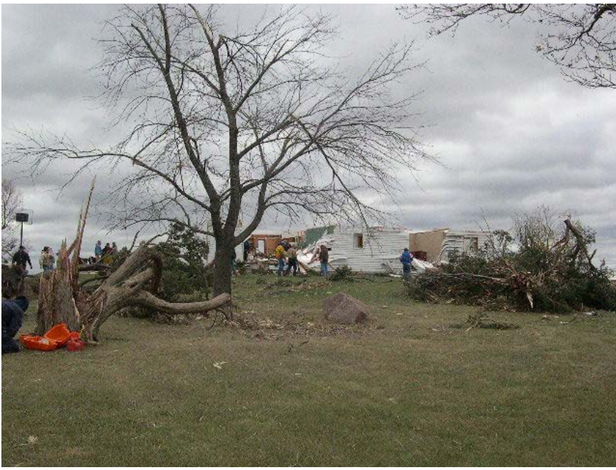
Home heavily damaged near 6 Avenue north of Pilot Mound in Webster county.
