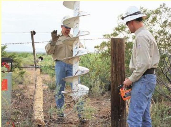
Utility workers repair power lines blown down during the August 4 severe thunderstorms at Boles Acres. (Michael Johnson/ Alamogordo Daily News)
