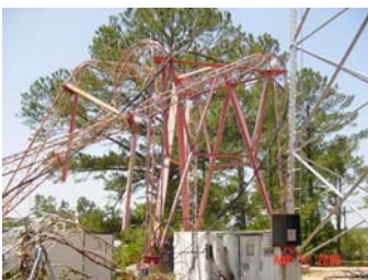
The remains of the Macon NWR tower after the 2008 Mother's Day storms.
