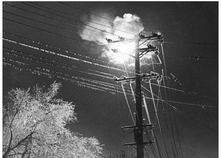
Wires shot out on a utility pole on Bridge Road - Monona Bruce Fritz
