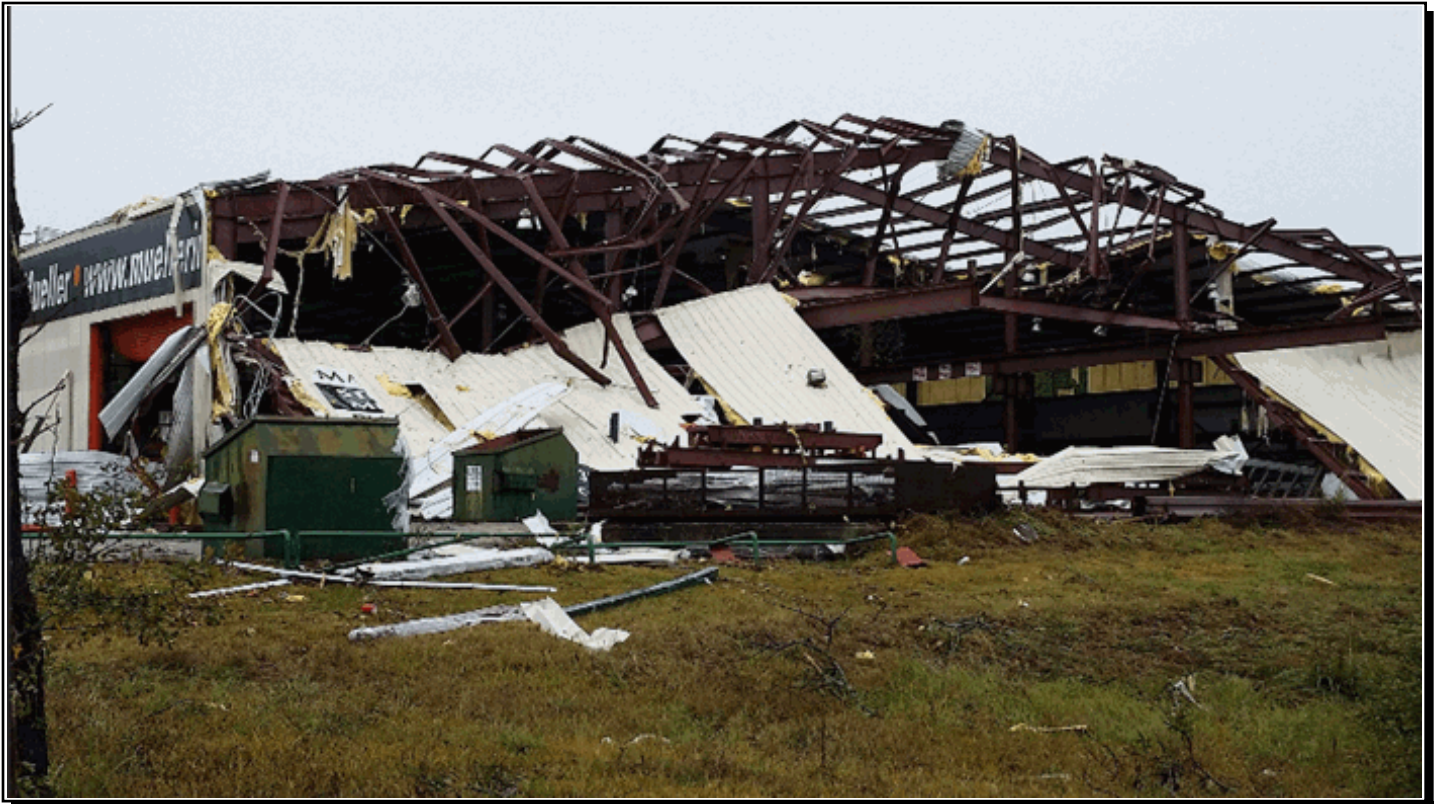
Tornado Damage north of Willis in Montgomery County, Texas
