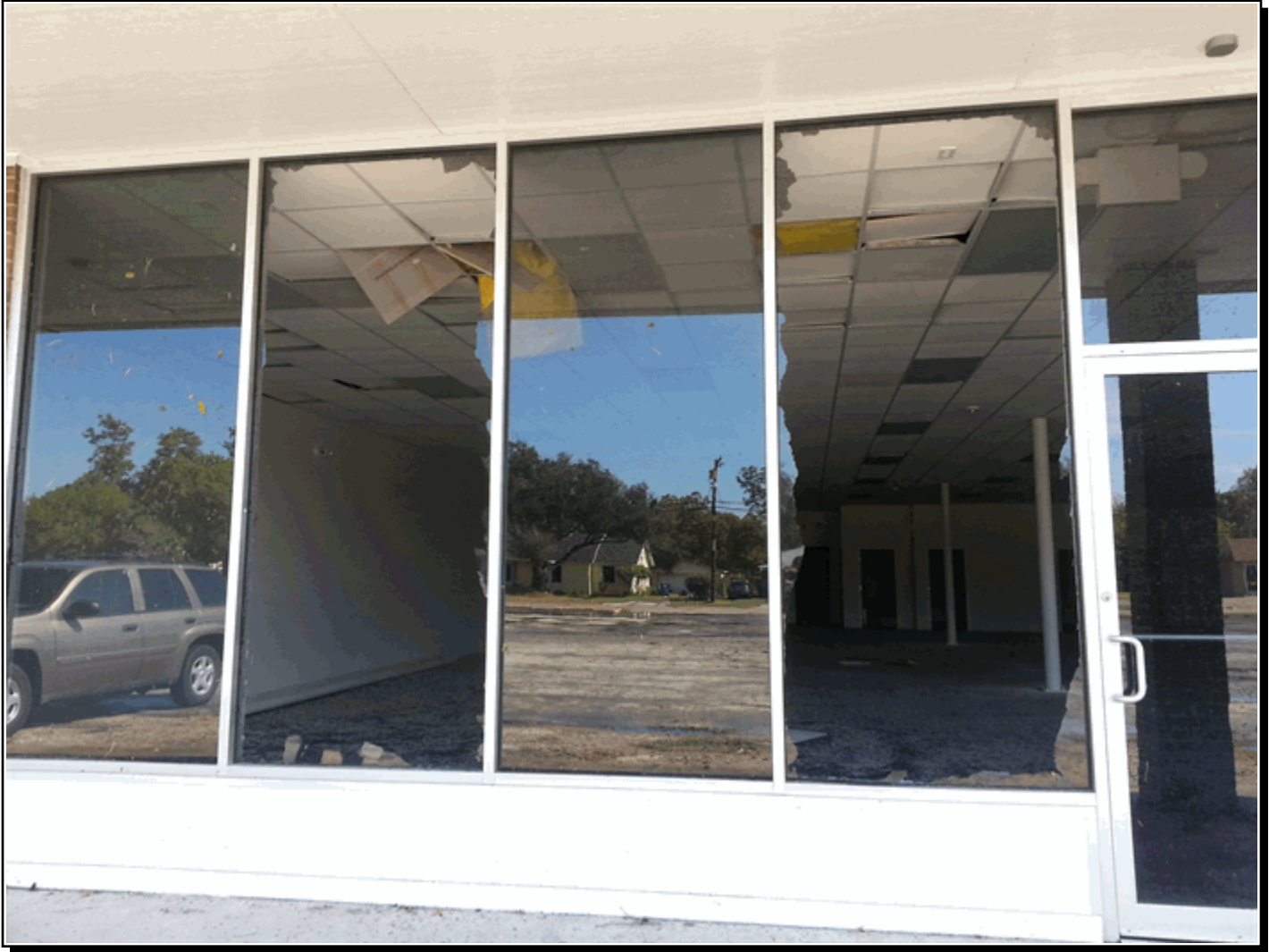
Commercial window damage in a strip mall across from the La Marque fire department.
