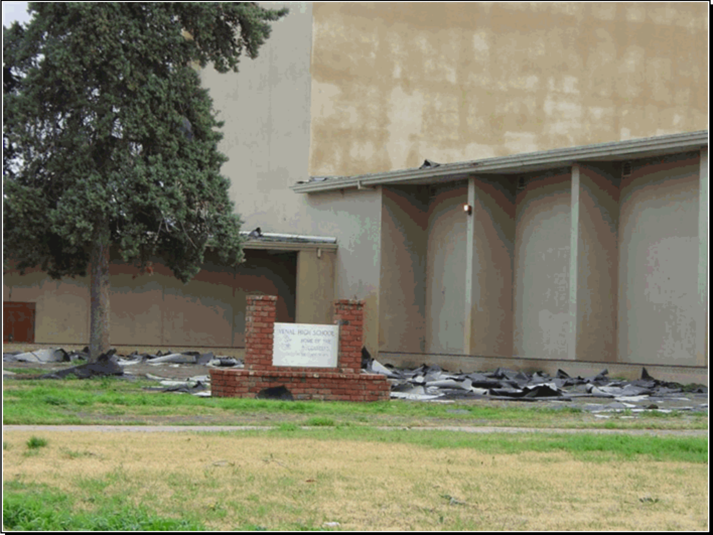
Widespread roof damage at Avenal High School. High winds were caused by a combination of strong large-scale winds and the local development of a mountain rotor cloud. Peak winds estimated at 70-75 mph. Photo courtesy CA Office of Emergency Services.
