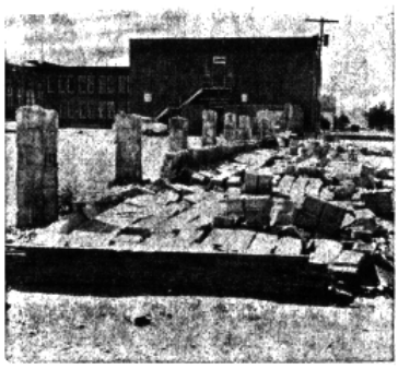
This cement block wall at the west end of the Morehead City High School athletic field was flattened Saturday night.
