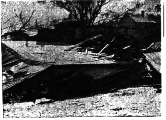
Helene lowered the boom on this house on Cedar Street, Beaufort. The walls collapsed and the roof settled directly on the foundation.
