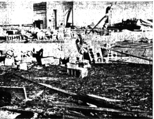
The Dainty Maid Bread Co. warehouse on the Atlantic Beach Causeway was leveled by the force of Helene's high winds. The large front doors blew open and the wind went through the cement block building, taking nearly everything with it.
