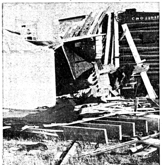
Thousands of dollars of damage was caused to the Freeman Wholesale Co. when the roof blew off between 3 and 3:30 p.m. Saturday. Rain then caused more loss by wetting the merchandise stored inside. Part of the concrete block wall collapsed on the west side, shown above, and landed on top of a box car.
