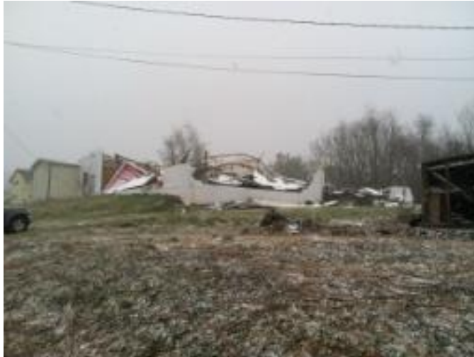
Warehouse building destroyed
