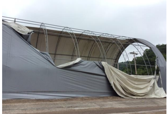
Salt Storage Facility Torn Cover
