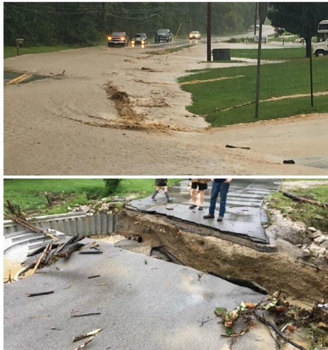
Significant flash flooding leading to a culvert on Dog Trot Road, west of Frenchburg, being
