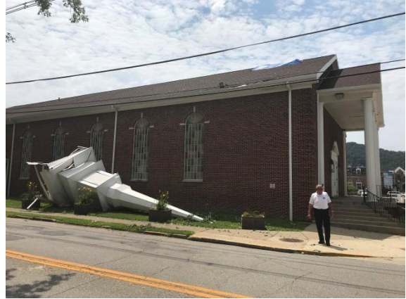
Church Steeple toppled from top of church in downtown Paintsville.
