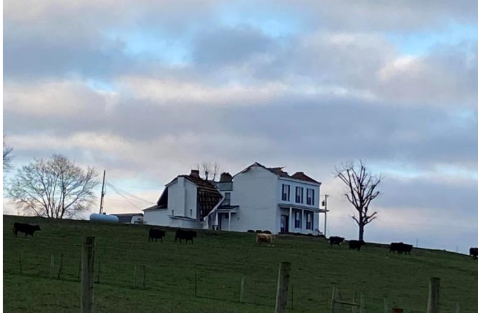
Roof blown off a farmhouse in Fleming County Picture courtesy of: Fleming-Mason Energy
