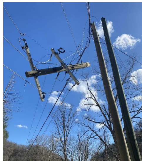
Power Pole snapped on Spurlock Creek- Floyd Co. Picture Courtesy of: Big Sandy RECC
