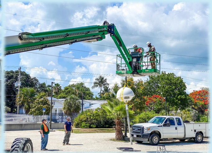
MROS installation crew begins to lift the new UHF antenna system to the tower.
