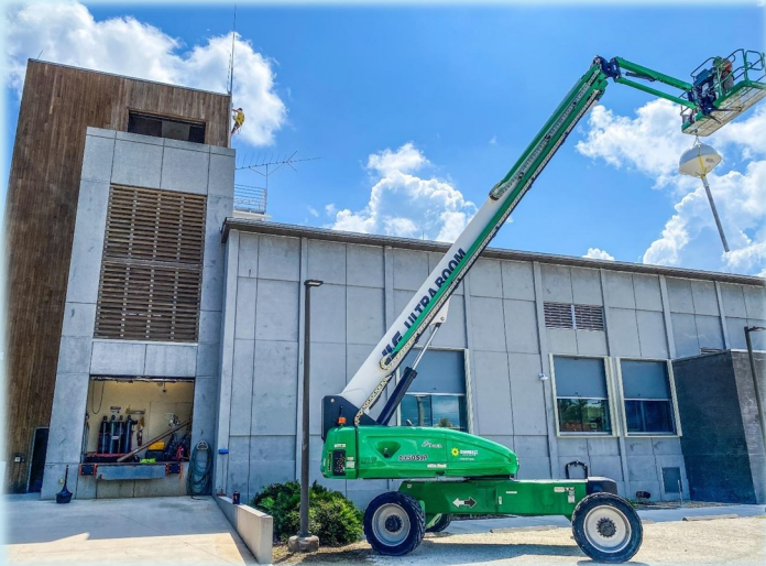
MROS installation crew hoisting the UHF antenna system up to the tower.
