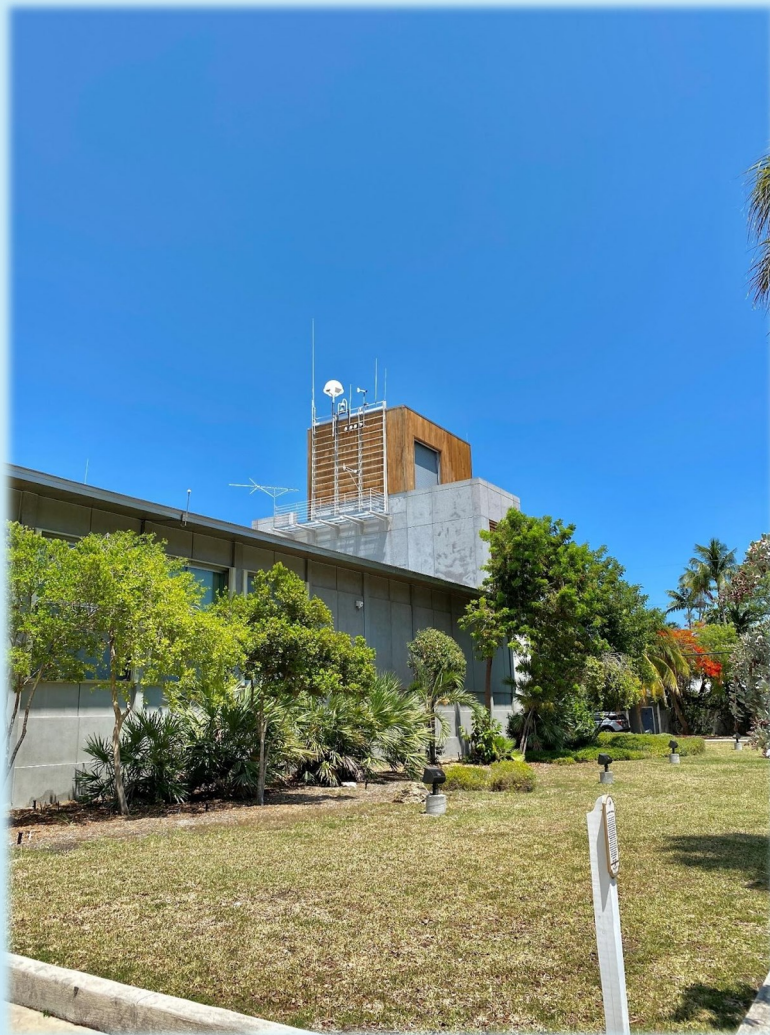
The new MROS UHF antenna dome installed on the Florida Keys NWS upper-air tower.
