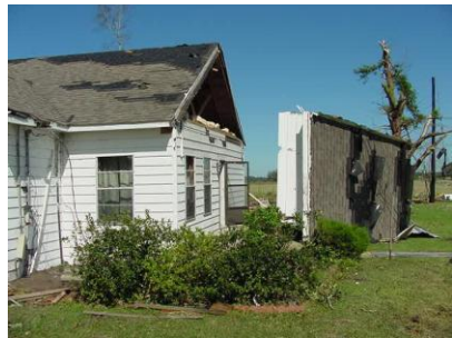
Tornado damage in China, TX
