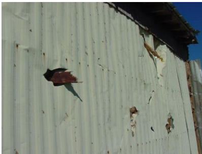
Tornado damage in China, TX
