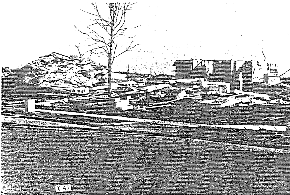
FIGURE 62. RESIDENCE. Exterior walls and the roof were blown away. The remaining room could have provided a shelter to the occupants.
