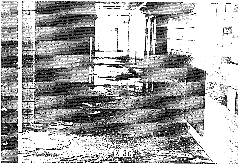
FIGURE 39. ARROWOOD ELEMENTARY SCHOOL, INTERIOR HALLWAY. The hallway sustained no damage and is free of flying debris. Pieces on the floor are acoustic panels of the hallway ceiling which became loose.
