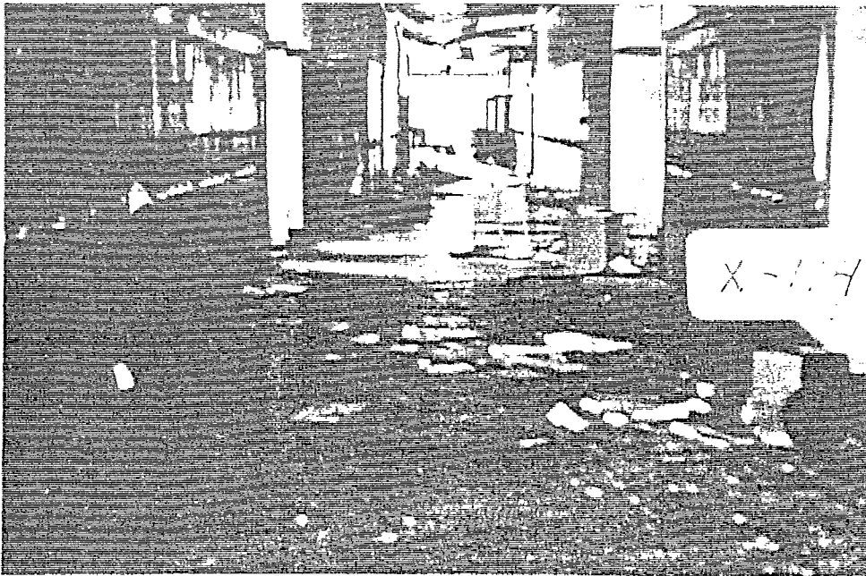
FIGURE 51. CENTRAL JUNIOR HIGH SCHOOL, INTERIOR HALLWAY. The second floor hallway was free of debris. This lack of damage and lack of debris was typical on all three floors.
