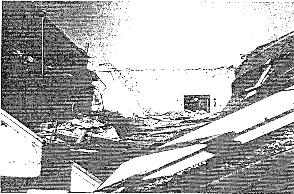
FIGURE 73. CHENOWETH ELEMENTARY SCHOOL. Progressive collapse of roof was precipitated by the toppling of an 8 ft incinerator chimney. Debris from chimney can be seen in background near wall.
