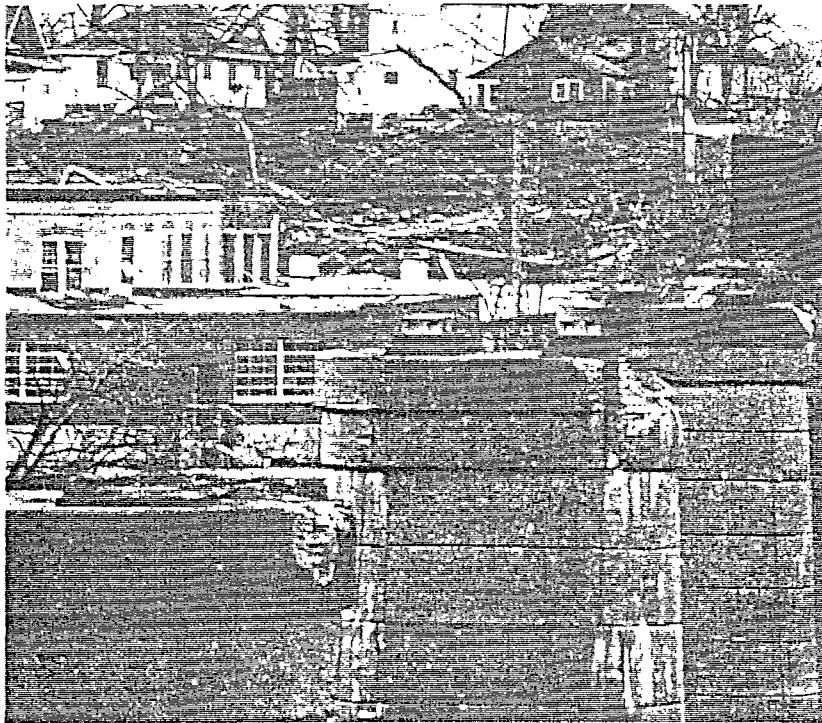
FIGURE 14. DAMAGED RAILROAD BRIDGE, MONTICELLO, INDIANA. Four spans, each with two 10 ft deep by 110 ft long girders, toppled into the river. (photograph courtesy J. J. Abernethy, University of Detroit-PASC)
