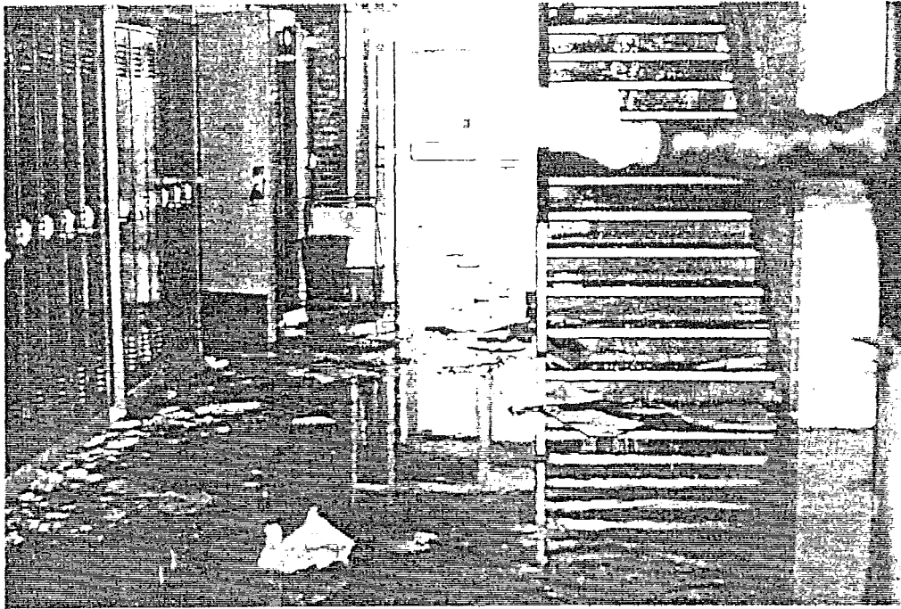
FIGURE 56. XENIA HIGH SCHOOL, INTERIOR HALLWAY. The first floor hallways were undamaged and were free of debris.
