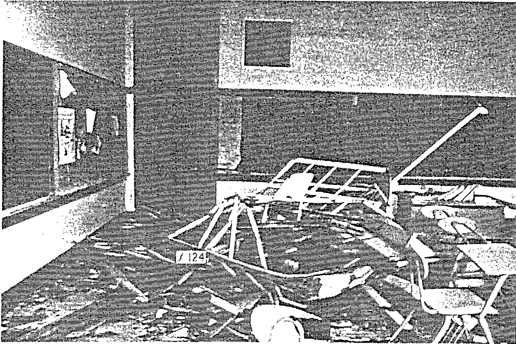
FIGURE 50. CENTRAL JUNIOR HIGH SCHOOL CLASSROOM. The second floor classroom contains a portion of a roof (approximately 40 sq ft in area) which flew in breaking the window frame. The roof and the window frame are visible.
