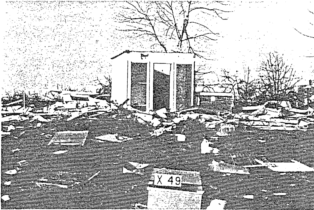
FIGURE 61. RESIDENCE. Roof has been uplifted. The interior walls remained intact.
