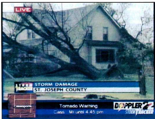
Fig. 6. Screen shot showing live picture of tornado damage in Crumstown, Indiana, as well as Tornado Warning information for Cass County, Michigan.
