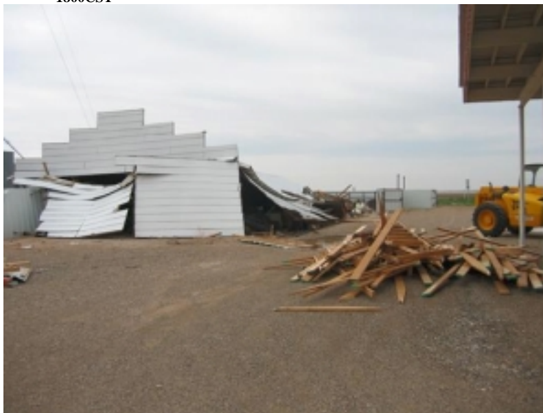
A heavily damaged industrial barn and scraps of lumber gathered by clean-up crews compose this scene following thunderstorms that produced significant wind damage in the Anton vicinity of northeastern Hockley County during the early evening hours of the 3rd. Damages there exceeded $400,000. Photo courtesy: National Weather Service - Lubbock, Texas.
