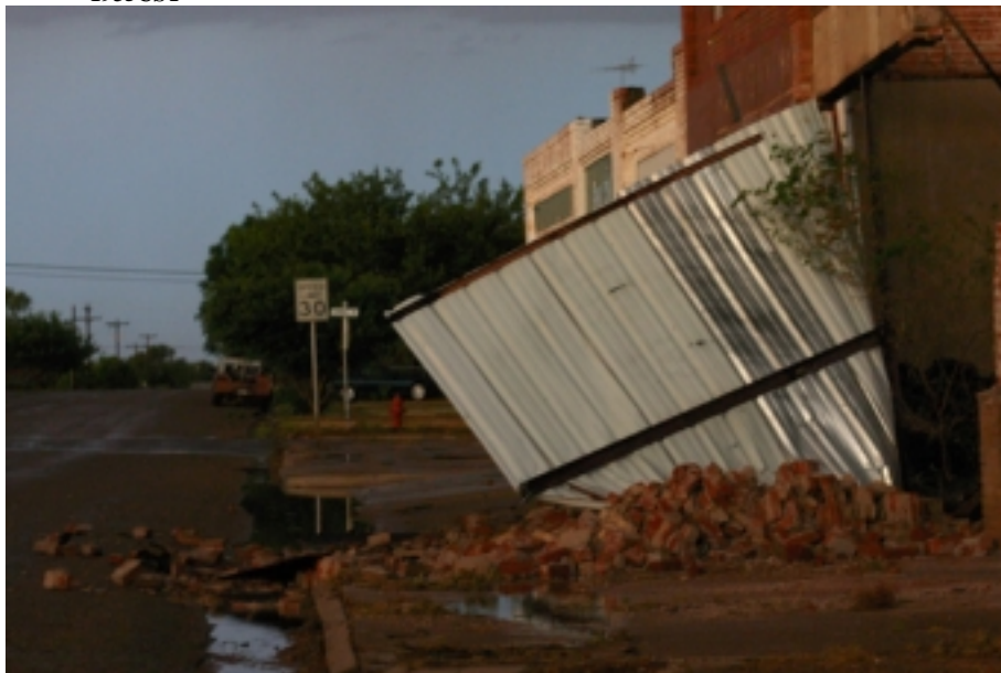
Damage to buildings in downtown Spur following a destructive downburst that resulted in two injuries. Photo courtesy: Debbi Ball - Spur High School - provided by KAMC-TV.
