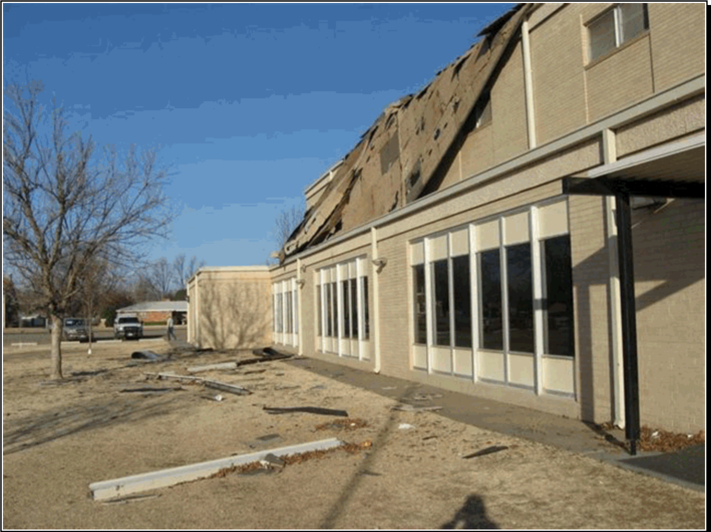
High winds in the wake of a frontal passage tore a large section off of the Memphis High School gymnasium in Hall County during the very early morning hours of the 21st. Photo forwarded by: Texas Tech University West Texas Mesonet.
