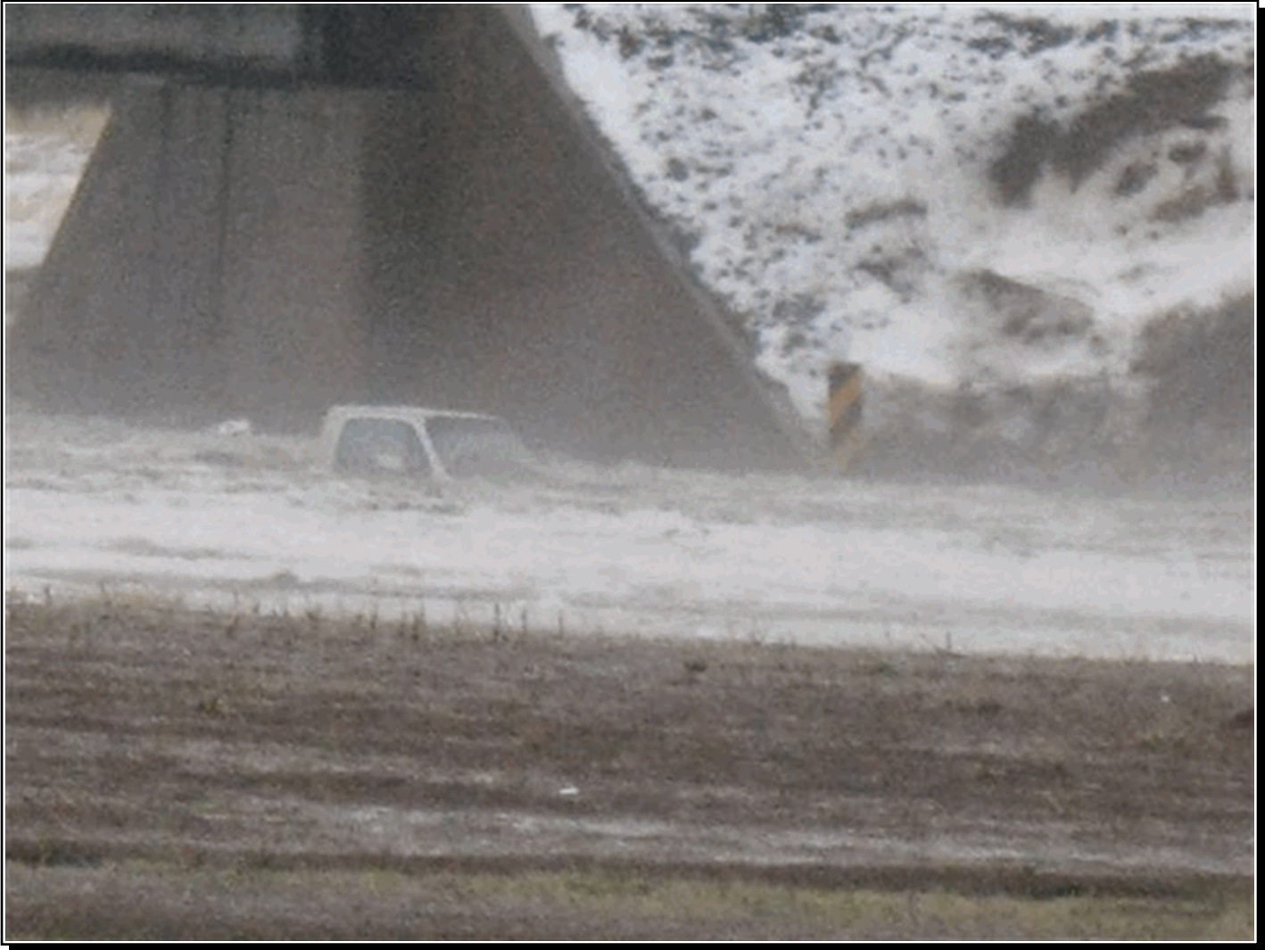
A combination of accumulating hail and heavy rainfall resulted in "ice jam-like" flooding along Interstate 27 between Kress and Tulia in Swisher County during the afternoon and evening of the 16th. Photo courtesy: Julie White - via KCBD-TV - Lubbock, Texas.
