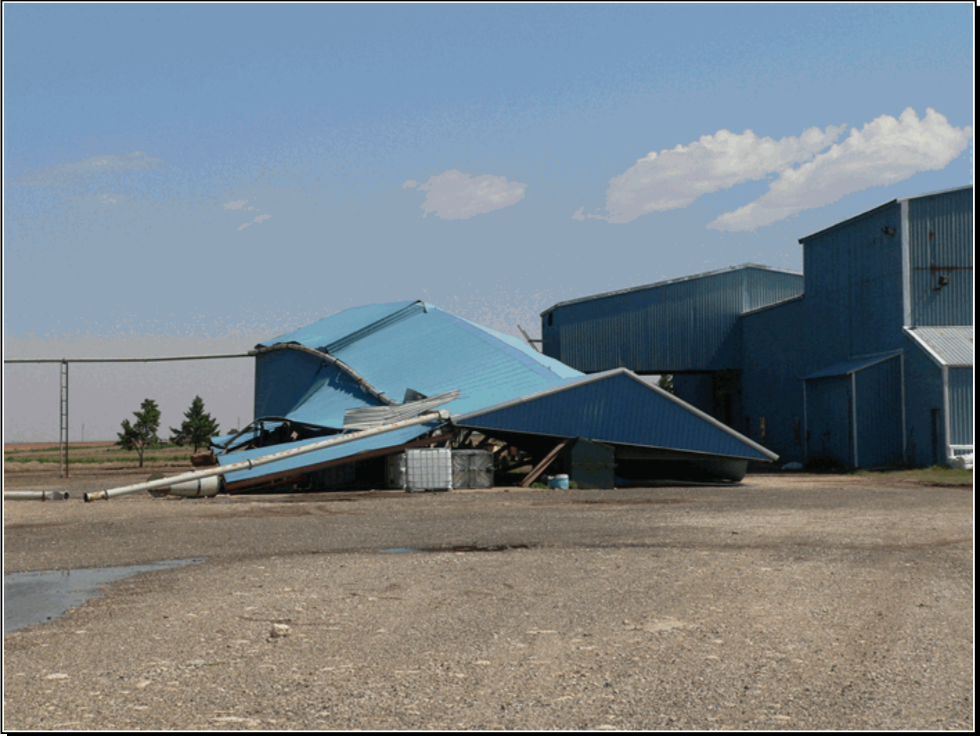
A large metal storage facility collapsed in severe thunderstorm winds at a cotton gin east of Brownfield, Texas, during the late afternoon of the 14th. Photo courtesy: National Weather Service - Lubbock, Texas.
