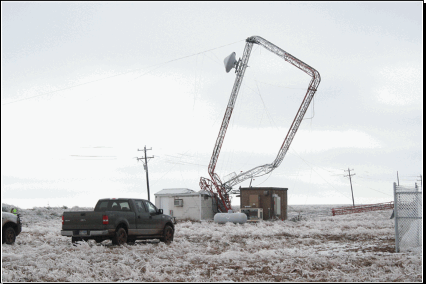
A radio tower collapsed under the weight of significant ice accumulations near Childress (Childress County) during a winter storm on the 28th. Photo courtesy: Ryan Mills - Childress Index - Childress, Texas.
