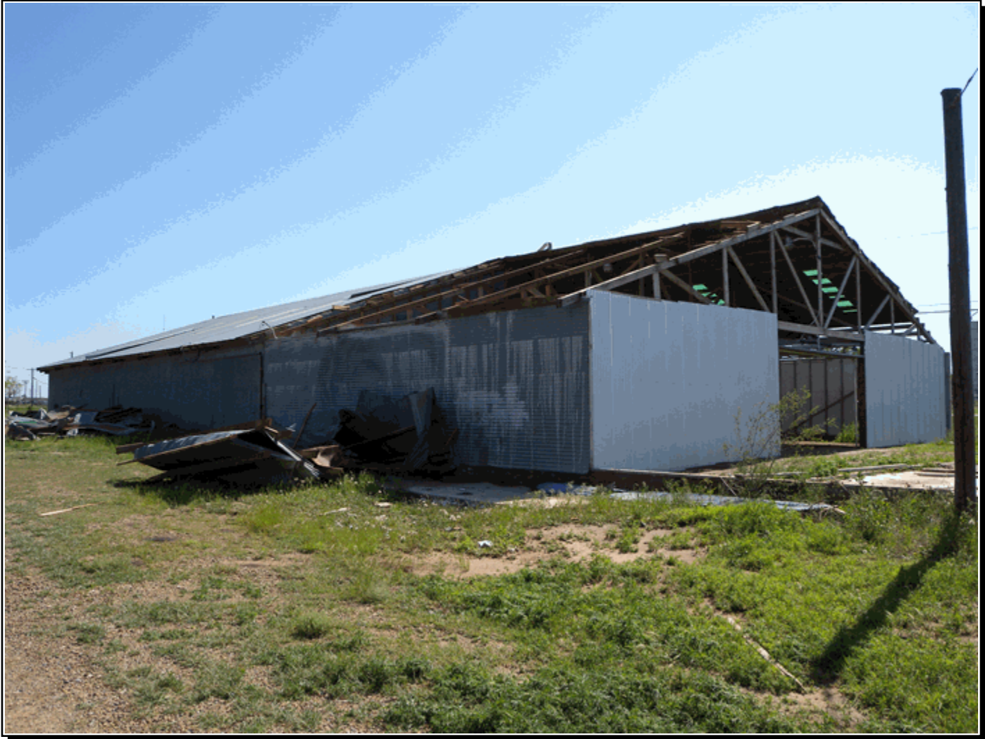
Thunderstorm winds removed a large section of roof from a metal barn in Floydada on the morning of the 17th, and resulted in other instances of structural damage in the city. Photo courtesy: Jody James - National Weather Service - Lubbock, Texas.
