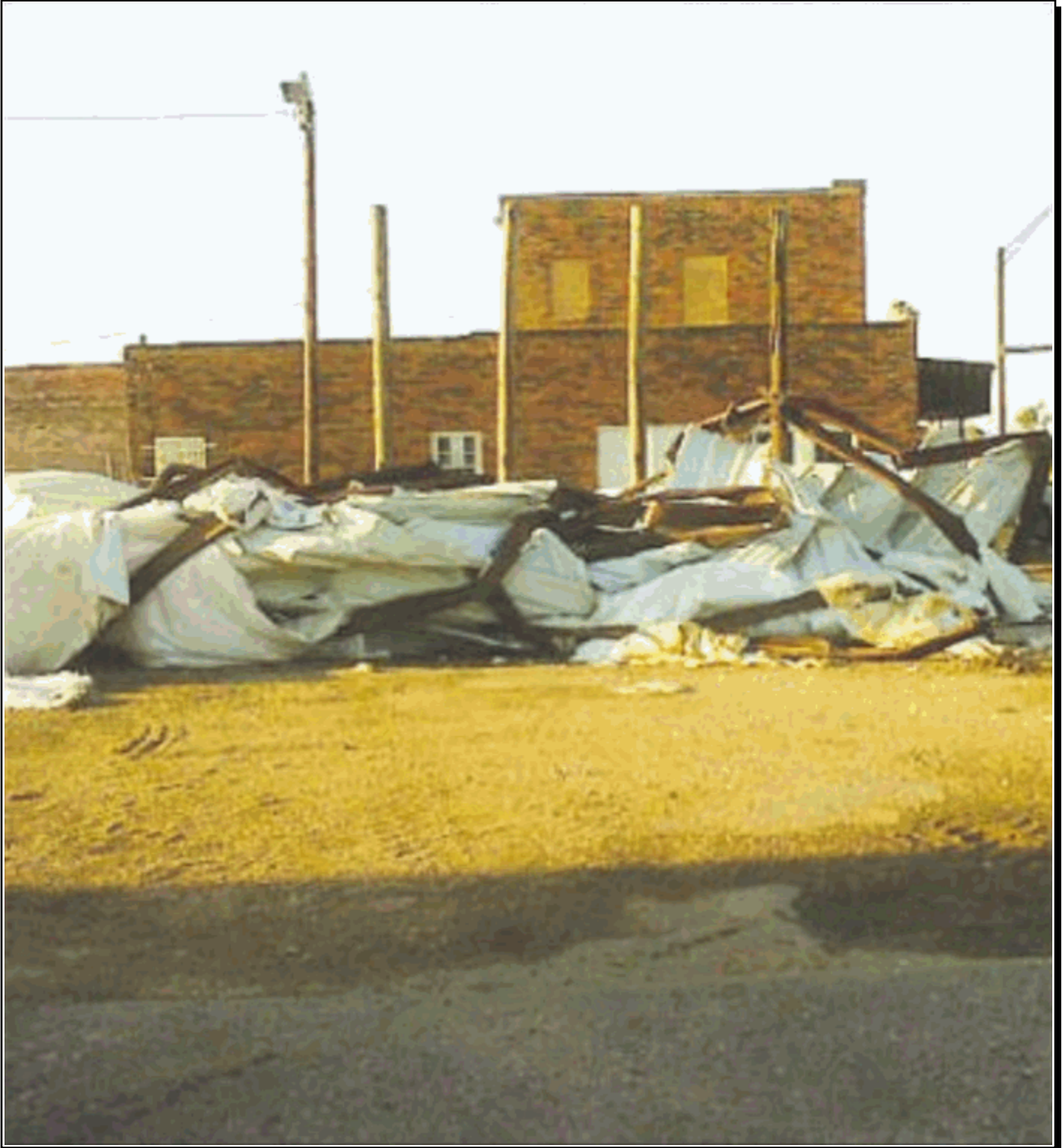
Thunderstorm winds caused extensive damage to the Estelline (Hall County) City Hall shortly before 18:00 CST on the 1st. Photo courtesy: Rene Miller via the Childress County Index.
