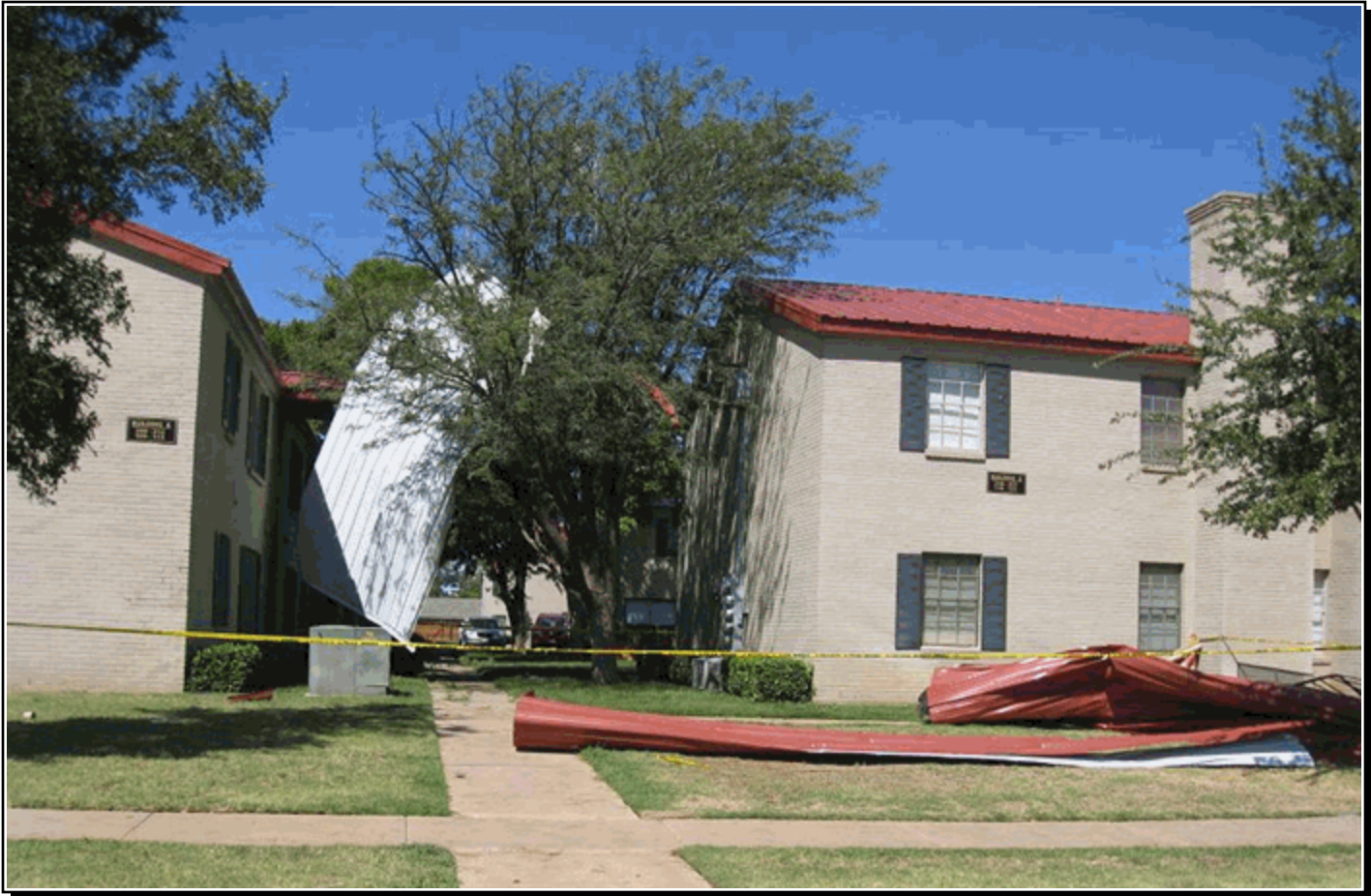
A roof blown off an apartment complex in west Lubbock after a downburst struck with winds between 60 and 75 mph. Photo courtesy of Steve Cobb.
