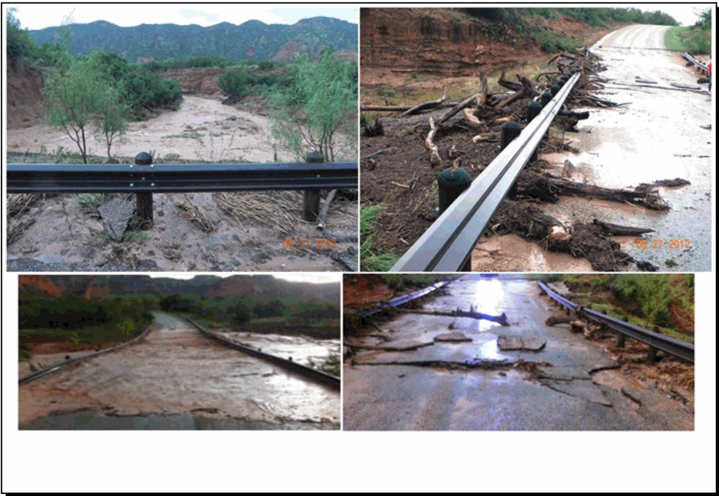
Photo collage of flash flooding at Caprock Canyons State Park. The floodwaters eroded outer sections of an asphalt road along a bridge. Photo credits: Caprock Canyons State Park.
