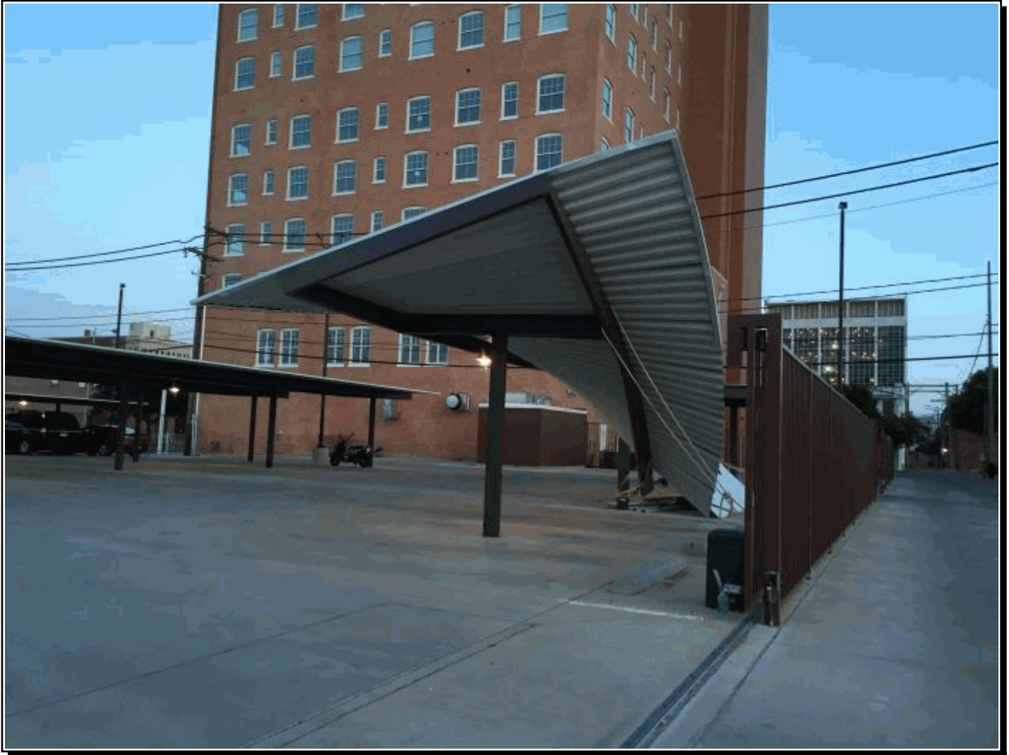
Wind damage to a parking overhang in Lubbock at 1204 Broadway Avenue. Photo by Caleb Holder, KCBD-TV news.
