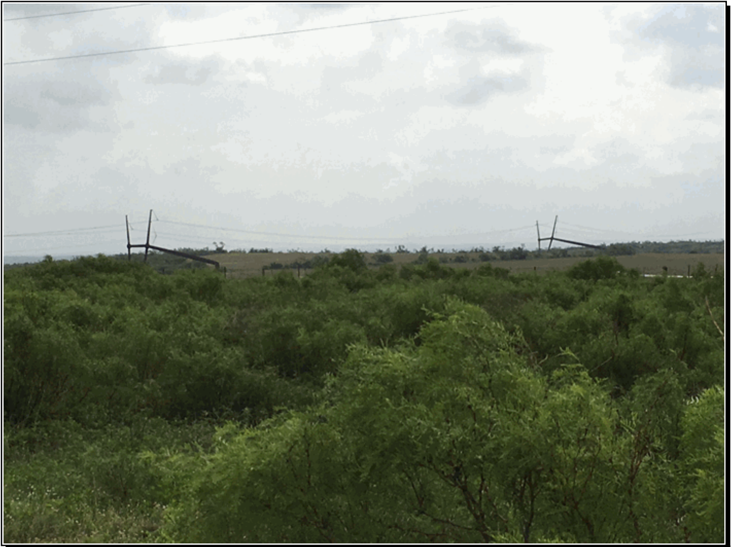
Photograph taken by an NWS post-storm ground survey. Several steel pylons supporting electrical lines were bent to the ground.
