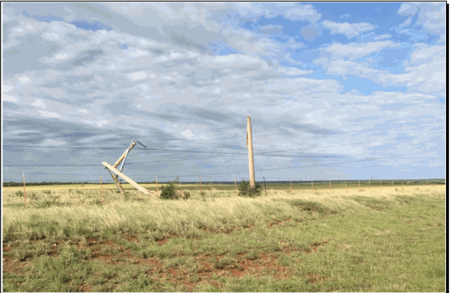
One of 16 power poles snapped along Highway 62 in northeast Childress County from a bow echo thunderstorm. Photo courtesy of Bill Ricks.
