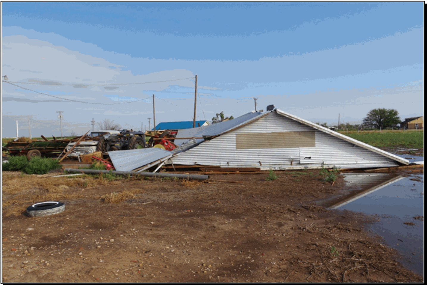
A large shed lost its roof during intense straight line winds of 80 to 100 mph that struck the community of Cone, TX on 9/17/2017. Photo from NWS Lubbock Storm Survey.
