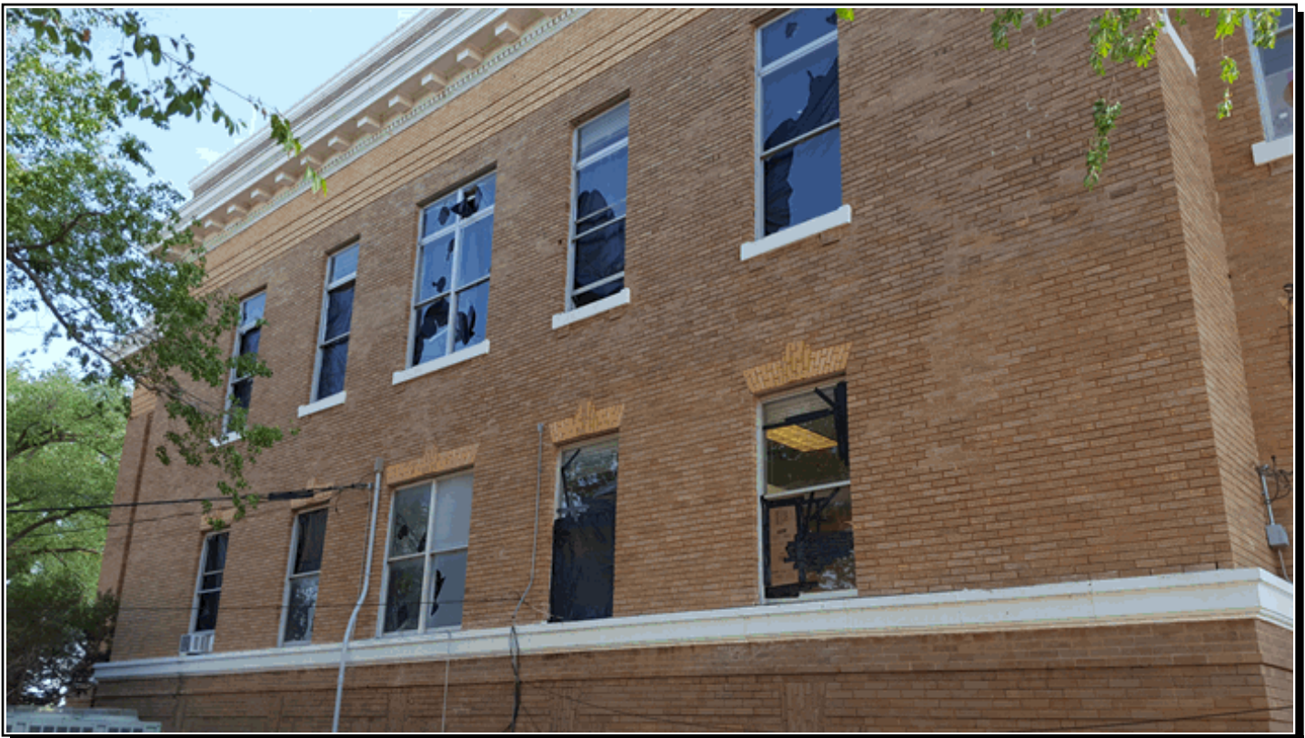
Photograph taken in Crosbyton of the southward facing portion of a building showing many broken windows. Photograph is from the NWS Storm Survey.
