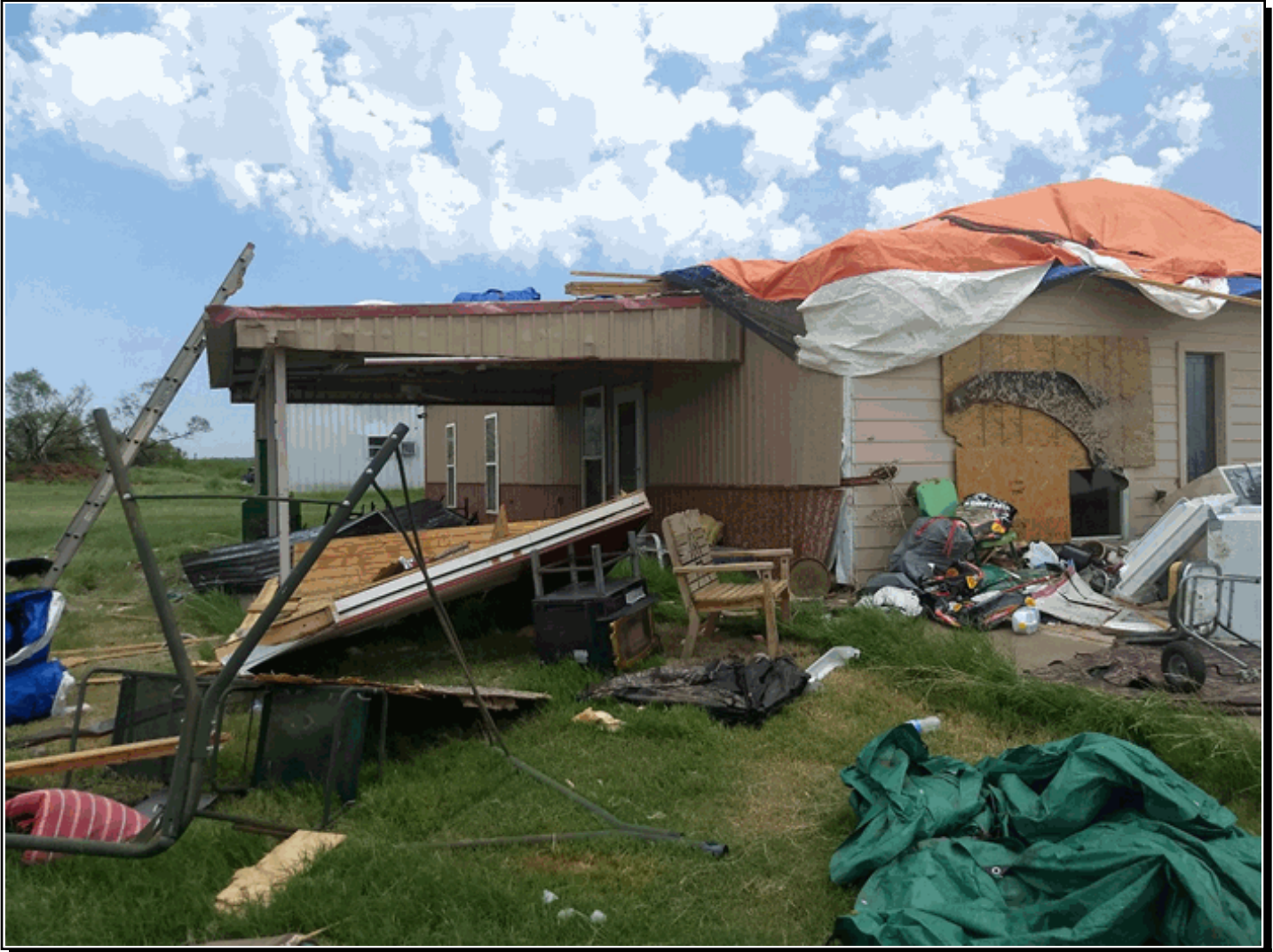
Photo of a heavily damaged home northwest of Estelline from a microburst. Photograph from a NWS storm survey.
